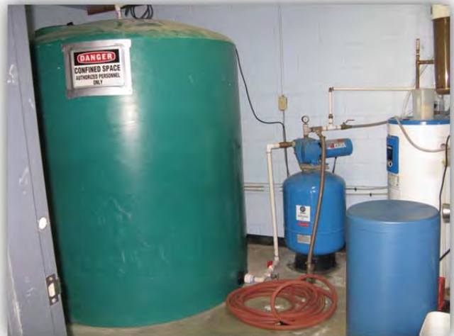
Rollo McClay Water Cistern
