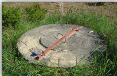
Rollo McClay Wellhead Cover in 2012
