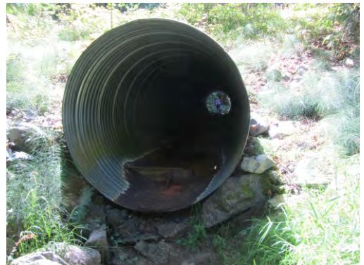
2,500 mm culvert under Wildgreen Way
