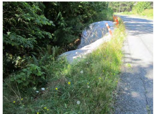
Slope failure of Allsbrook Road
