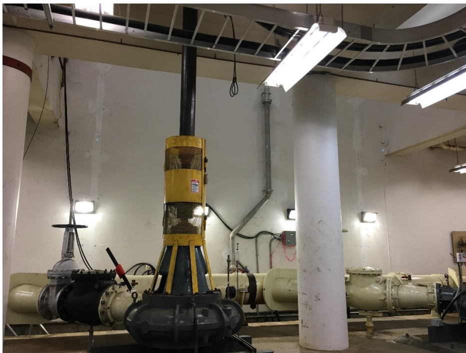
Figure 4-2 Piping Not Restrained
