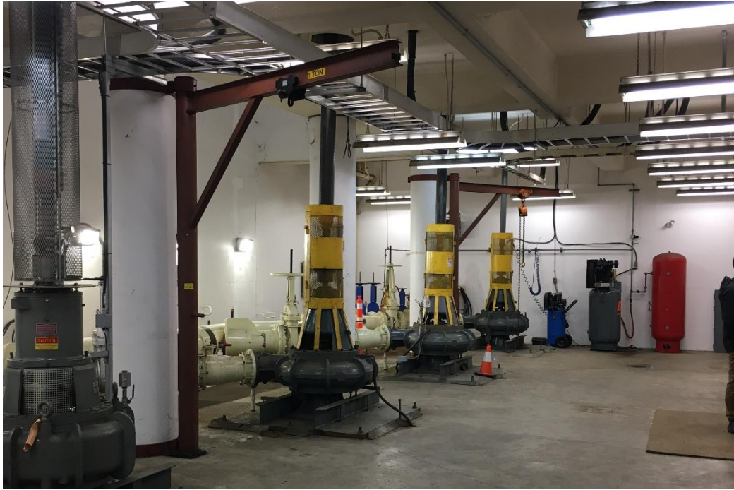
Figure 4-3 Lack of Seismic Restraints on Swing Arm of the Cranes
