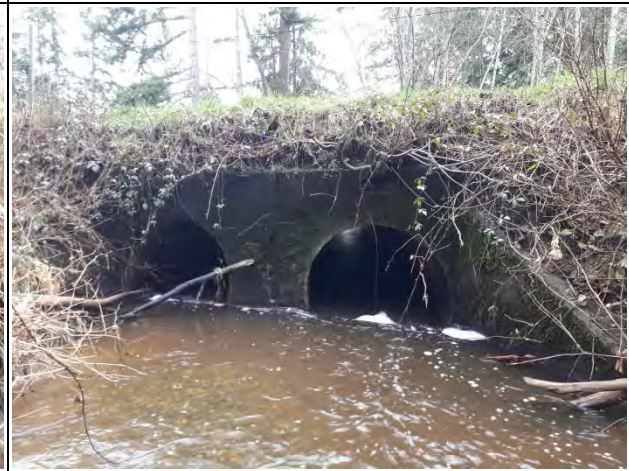
Photo 4: Facing downstream, showing the inlet of the dual-culvert crossing of Morningstar Creek at Highway 19A.
