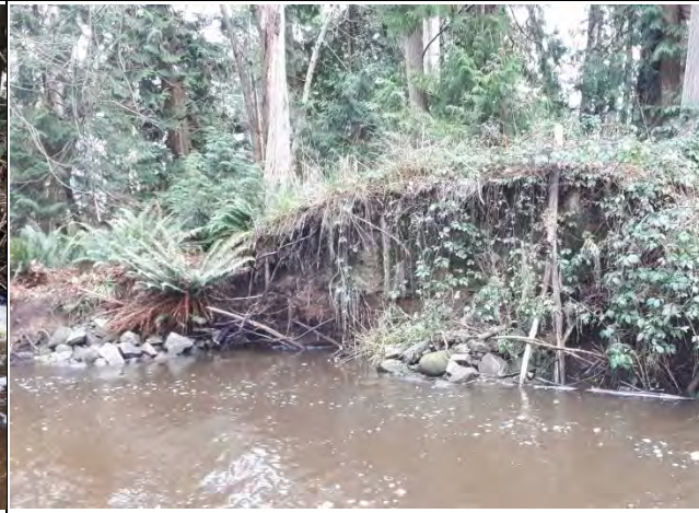
Photo 8: Facing the right downstream bank, showing two piles of angular stone placed against an eroding bank, likely intended to minimize further erosion.
