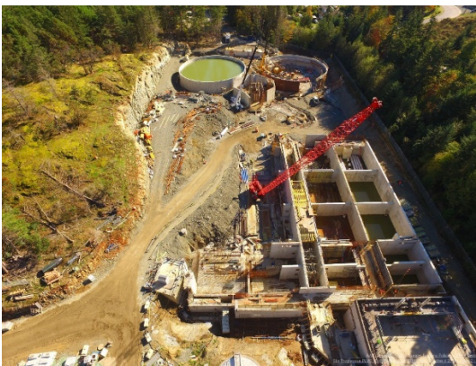
Photo left: Secondary treatment area – bioreactors and clarifiers
