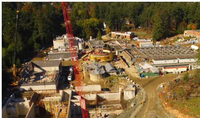
Photo right: Primary treatment and solids handling area
