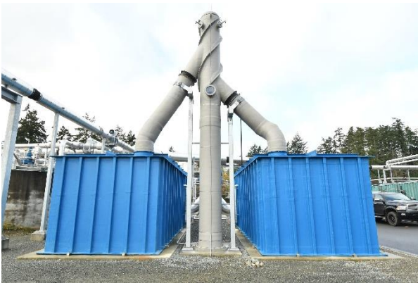
Odour Control Biofilter
