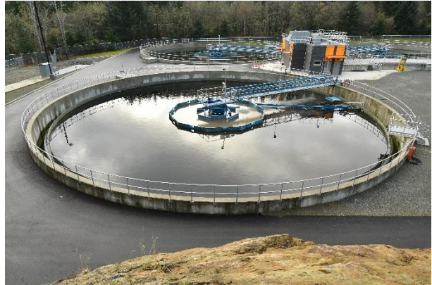
Secondary Treatment Clarifiers
