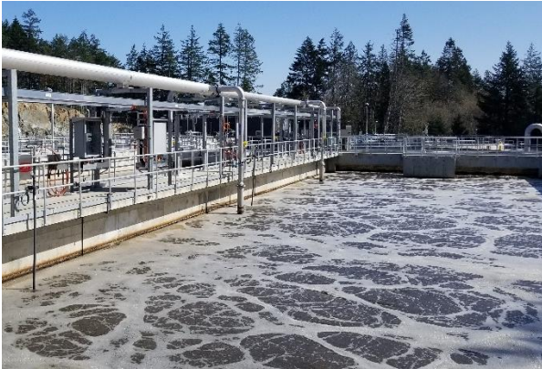
Secondary Treatment Bioreactor
