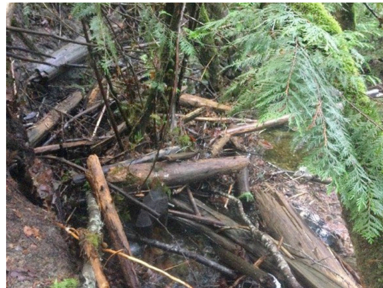
4.) R13 – Wolf Creek plugged culvert
