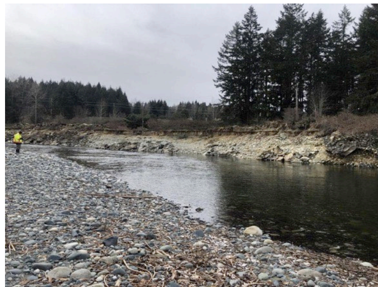
6.) Pool 2 – also showing LB erosion under trail/powerline
