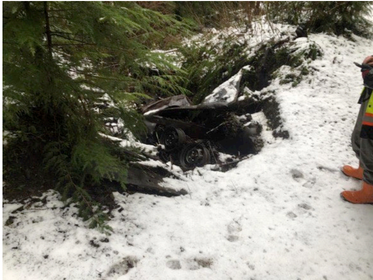
7.) P4- Plugged culvert along rail grade with old car body debris
