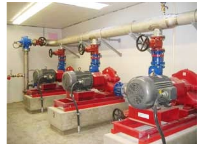
Figure 1.2.1. B) Groundwater pumping system for the Town of Qualicum Beach (courtesy of the Town of Qualicum Beach).
