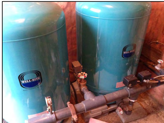
Pressure tanks in the pump house
