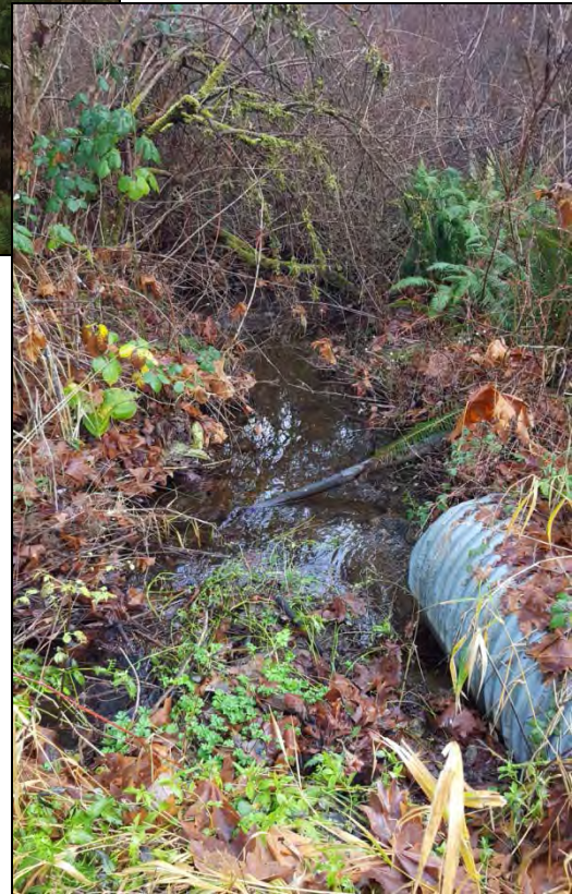
Photo 3. Showing the east side of the culvert crossing where it drains into the wetland area.
