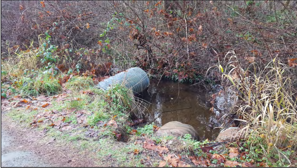
Photo 1. Showing the west side of Berkshire Road where Westglade Brook culverts are located connecting two wetland areas.
