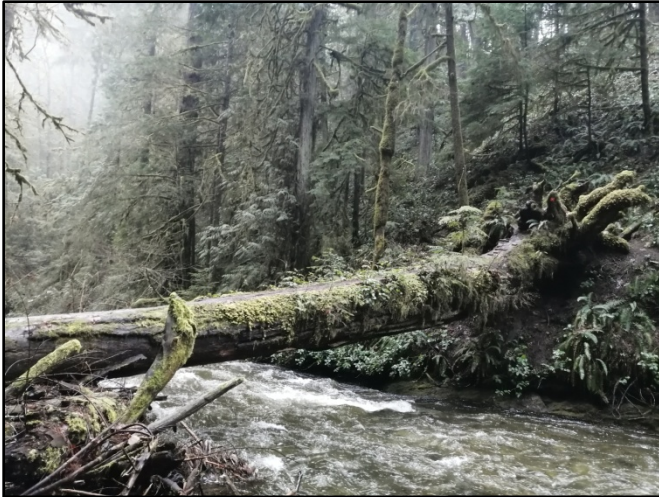
Photo 5: The fallen log crossing as seen from the toe of slope on the north side of Benson Creek. This will be replaced by a proposed truss bridge.
