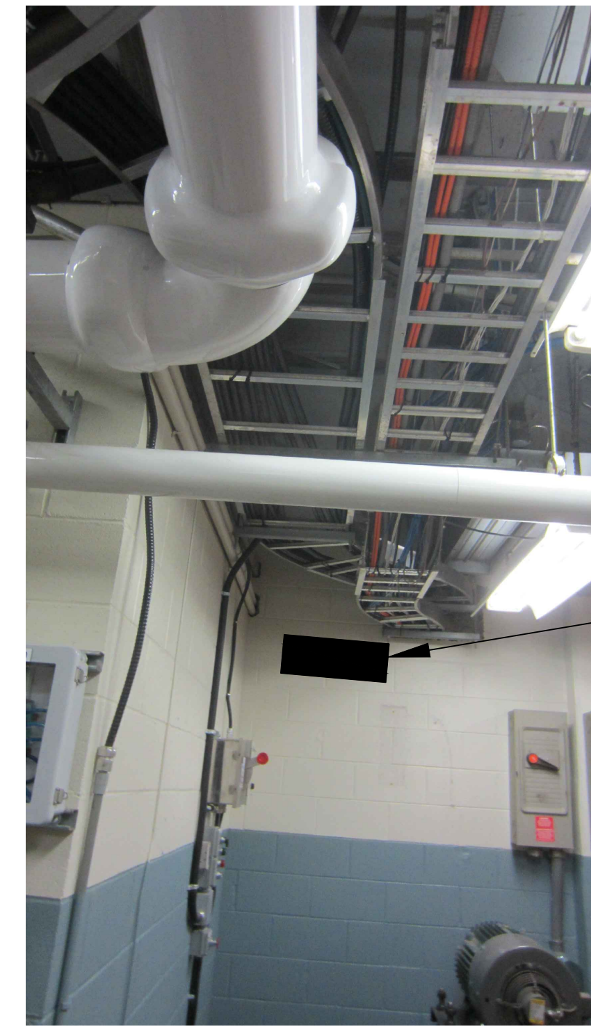
IMAGE 1 - CABLE TRAY TO ELECTRICAL ROOM (APPROX.)
