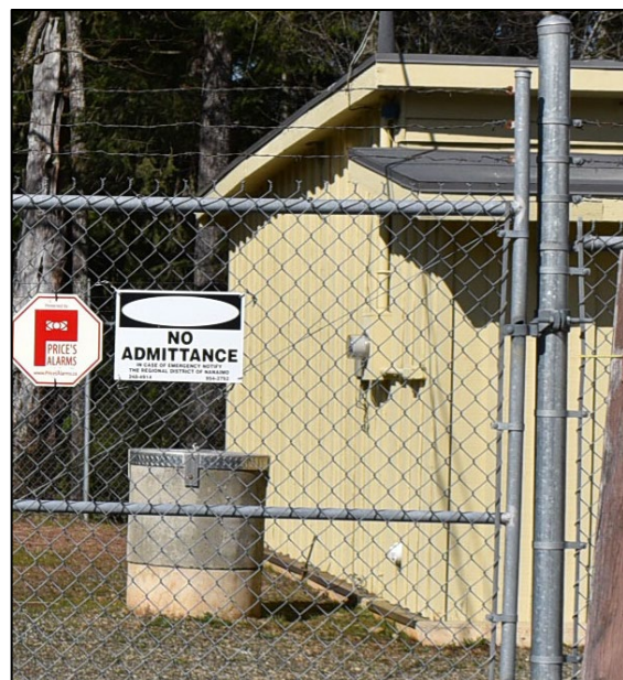
Melrose Well and Pumphouse
