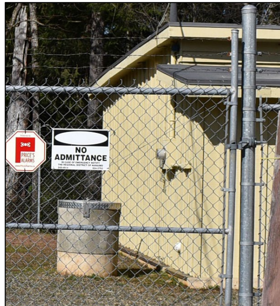
Melrose Well and Pumphouse
