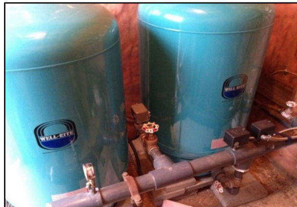
Pressure tanks in the Westerne Heights pump house
