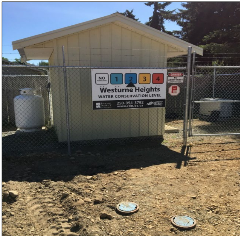
Westurne Heights Pumphouse and Buried Cisterns
